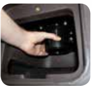
"Hands dry", large drain protected from the cold by a double-walled cover.
